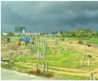
Piling works on the 'Entrepreneur Hub @ Pulau Li Hua' project in progress.
